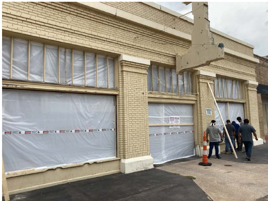
Figure 11: 1149 N. 2 nd St. Window Casings (Before)
