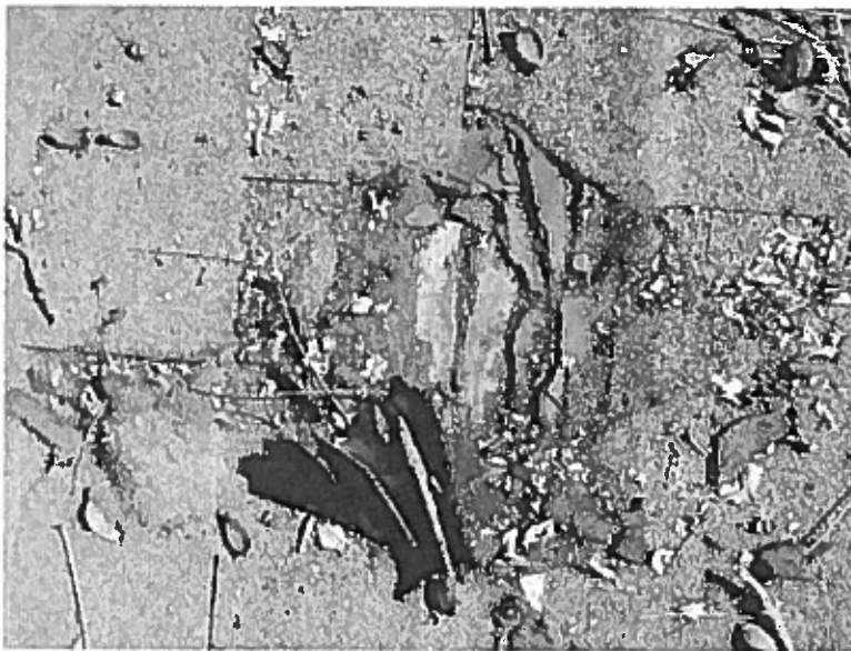
Figure 8. Roof damage with possible underlying structural damage.
