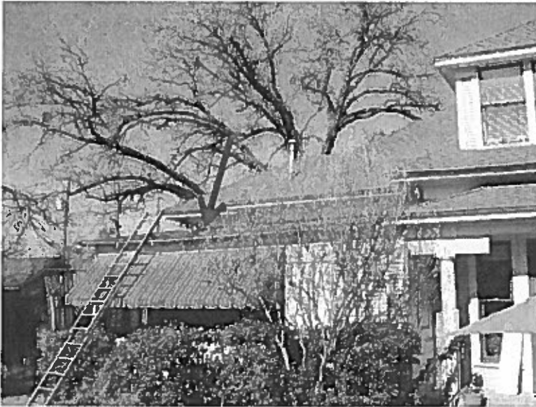
Figure 10. Deflection visible between lower eave and upper ridge of porch roof.
