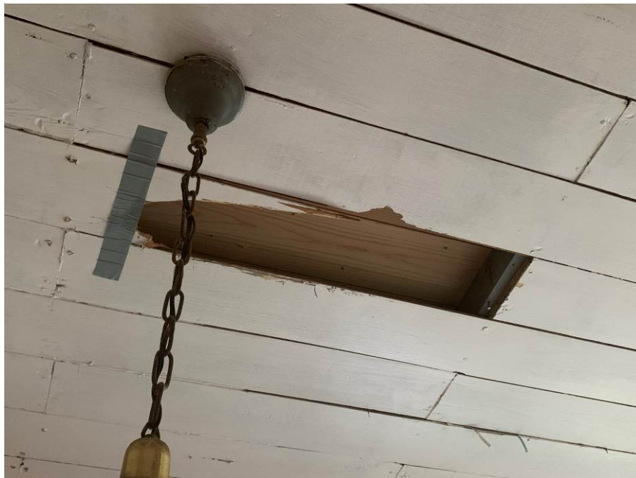
Figure 9: Porch interior view of damaged roof
