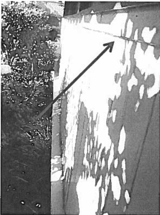
Figure 12. Inward bow in wall of porch.
