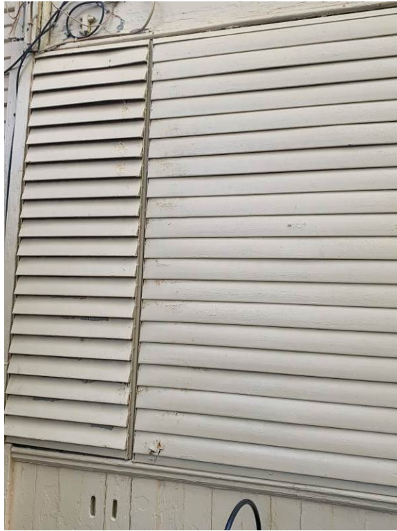
Figure 5: Rusted shut metal shutter siding
