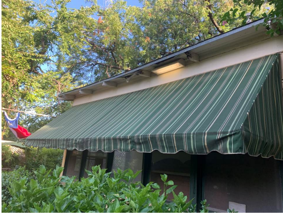
Figure 4: View of damaged porch
