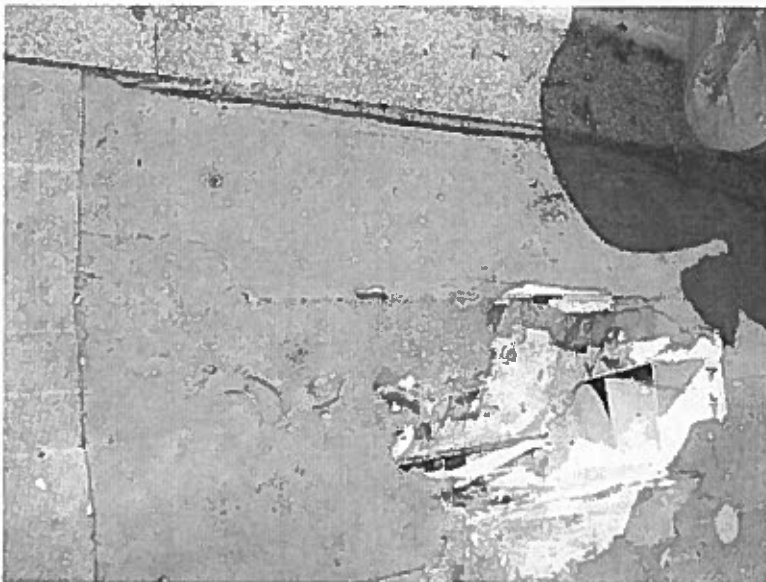
Figure 4. There were two layers of felt underlayment with the bottom layer hot mopped (due to the low slope of the roof).
