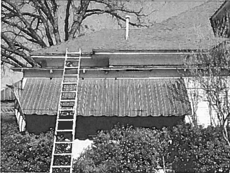
Figure 9. Deflection in eave of porch roof below damage (approximately at ladder).
