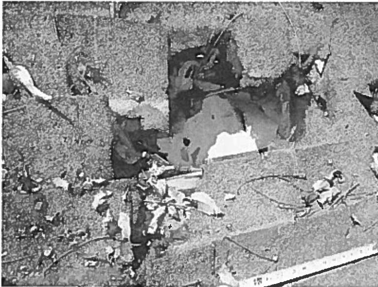
Figure 3. Tree damage penetration through roofing and roof sheathing (white duct tape is on the ceiling surface).
