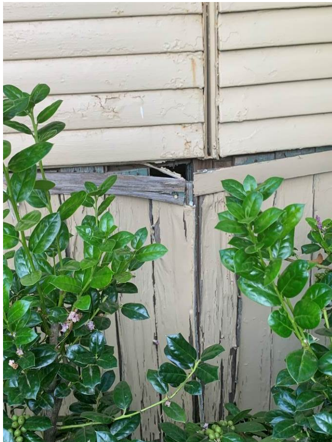
Figure 3: Damaged wood siding
