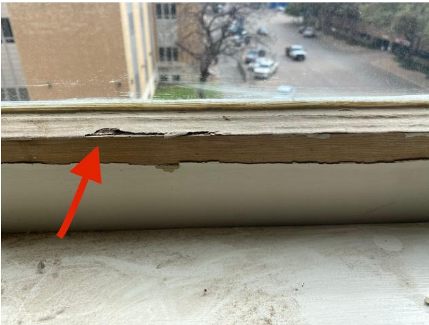
Figure 6: Deteriorated paint at base of interior of window
