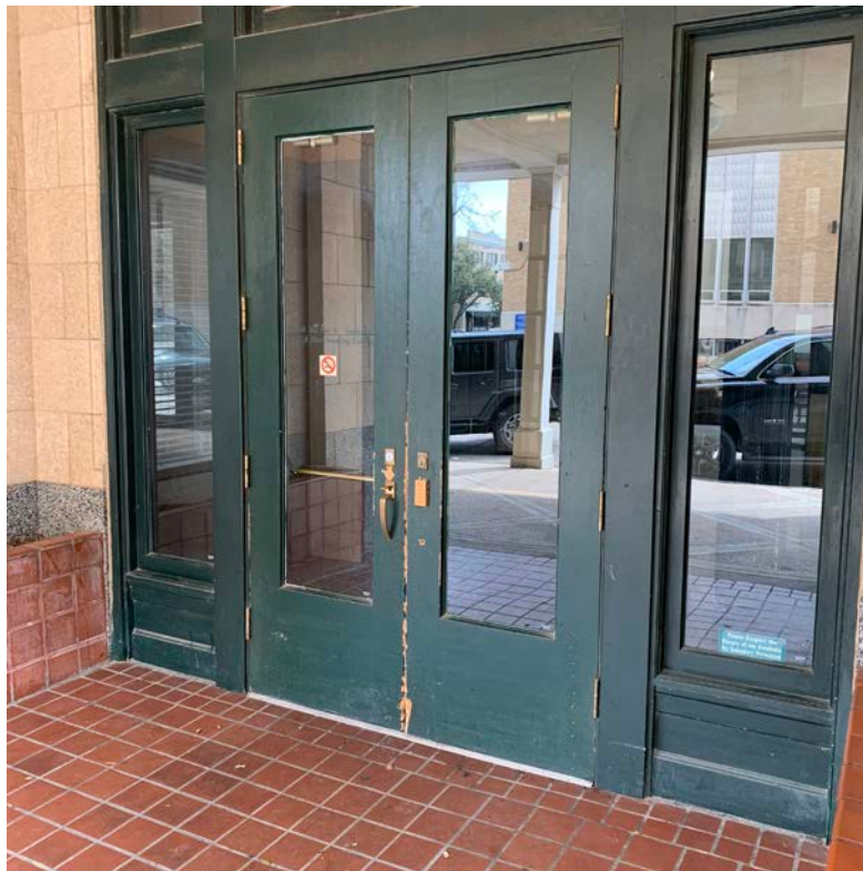
Figure 9 & 10: Damaged front double doors
