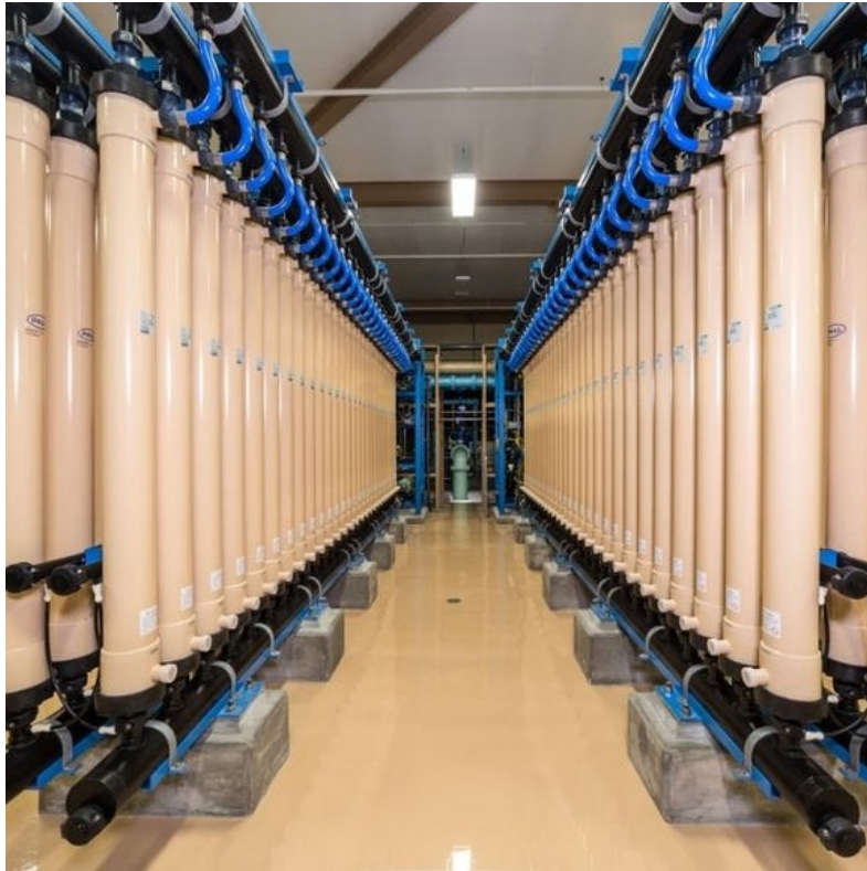
Microfiltration Rack w/ Modules
