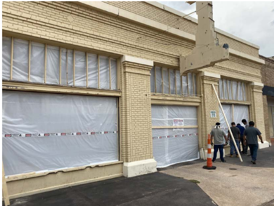
Figure 11: 1149 N. 2 nd St. Window Casings (Before)
