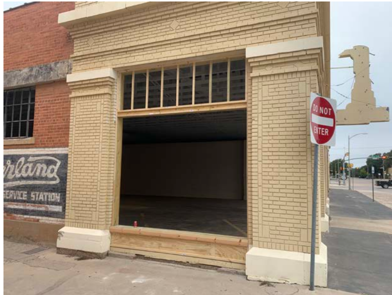
Figure 4: 1149 N. 2 nd alley Store Front Window Casing
